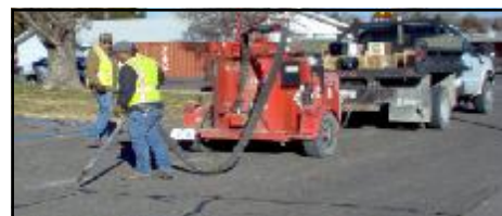
PW Dir. Steve Ferland and Steve Homburg work on crack patching by Spruce Villa.
